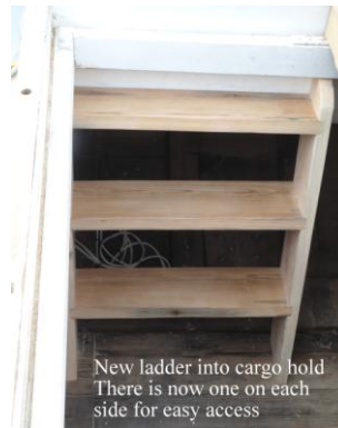
Boards are screwed onto the frame. Later they will be cut to form five easily removable hatch covers
